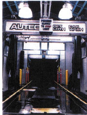
AUTECH helped make the clear car wash possible with its equipment.
